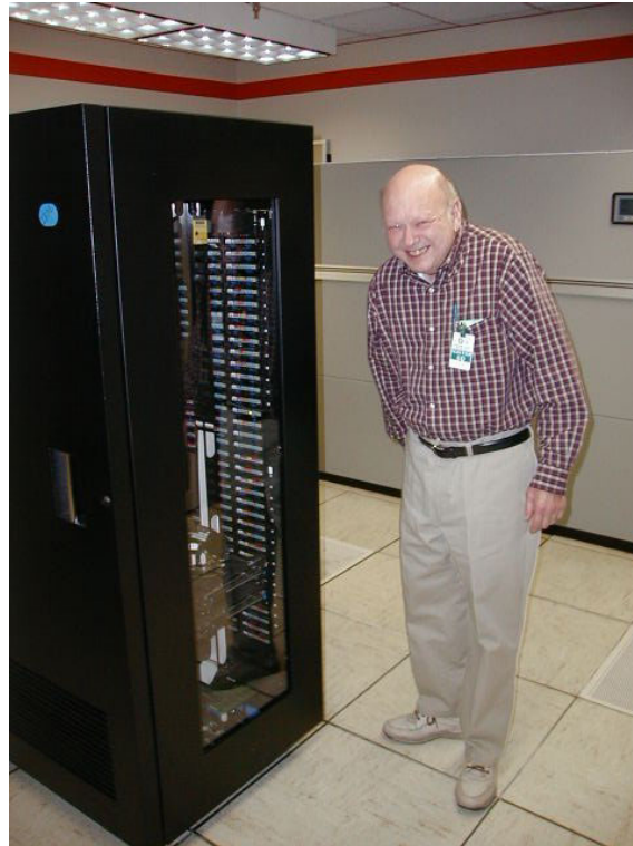
Jim Snyder at a nearby Data Center September 30, 2002
